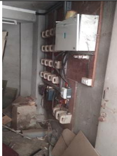
Meter Cabin with Waste Dumping Old Technology Used
