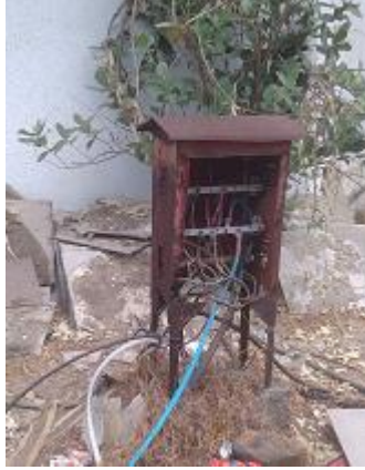
Damaged Feeder Pillar
