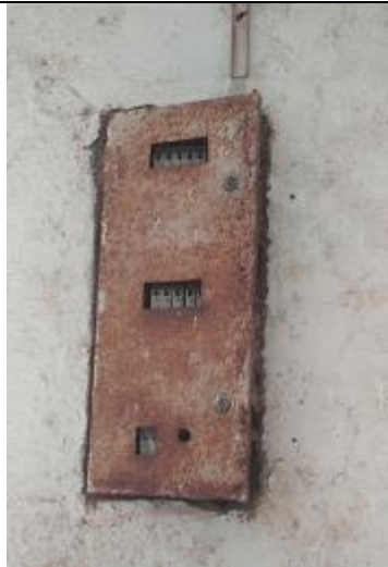
Old Risky Installations
