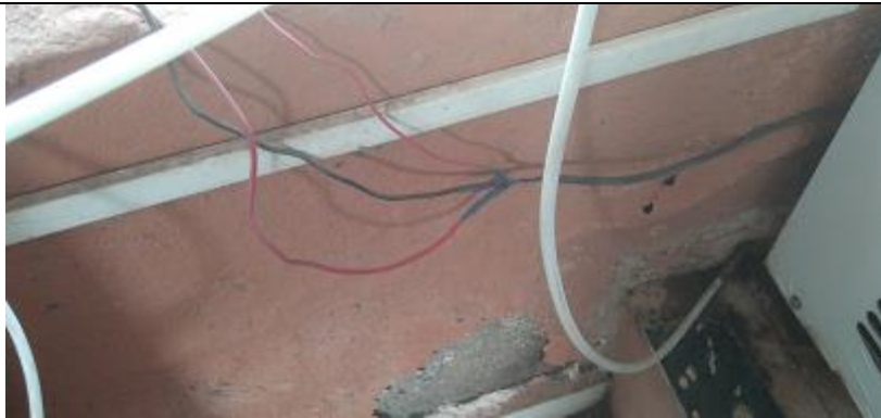
Non Insulated Portable cables
